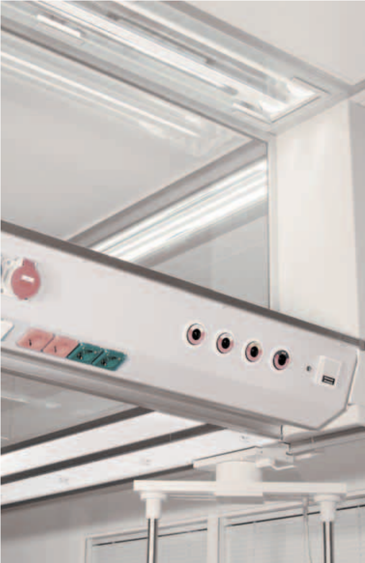
Media bridge: System "Modultechnik", with customized equipment and fittings
